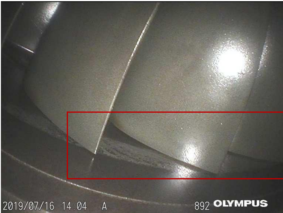
Picture 14 : light rub of free turbine shroud, at free turbine blade tips (red rectangle).
